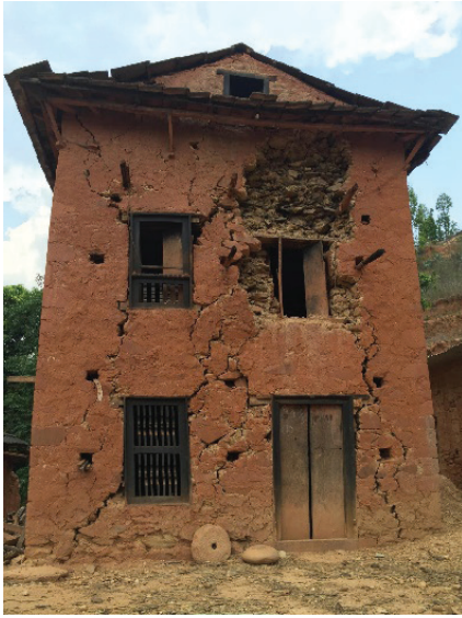
Figure 5. Out of plane damage in transverse walls including delamination in attic wall
