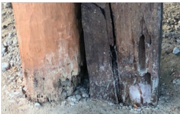
Figure 14. Deterioration of timber member at the base
