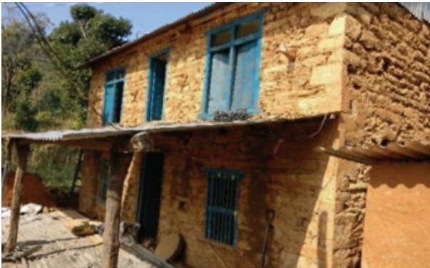
Figure 10. SMM house with rubble and high mortar-stone ratio
