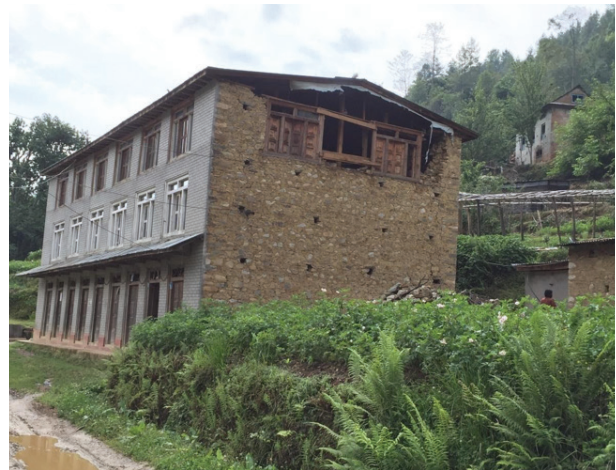
Figure 4. Collapse of gable walls, sometimes also destabilizes the wall below
